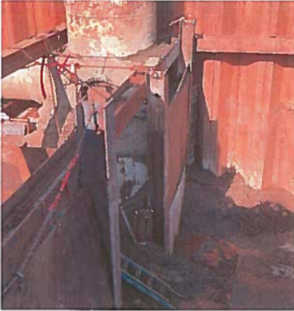
Slurry was poured between existing manhole structure and shoring plates to stabilize the foundation of the manhole after undermined soil was observed.
